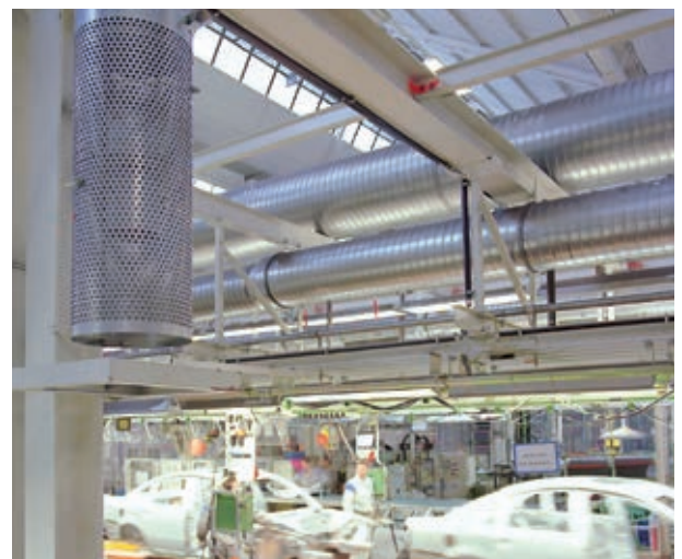
Fig. 16: Circular displacement outlets in car manufacturing halls
