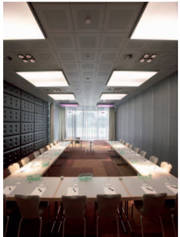
Fig. 5: Adjustable radial outlet in the meeting room of a hotel
