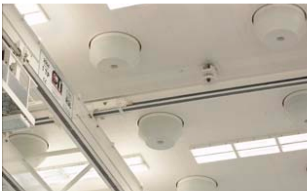
Fig. 1: Conical displacement outlet installed in the ceiling of a 26 m high hall
