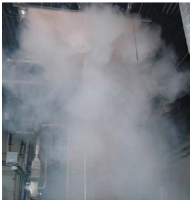
Fig. 6: Cooling mode with air outlet volume flow rate of 695 l/s [2 500 m³/h] and \Delta\vartheta_K = -5 K from 8.2 m height
