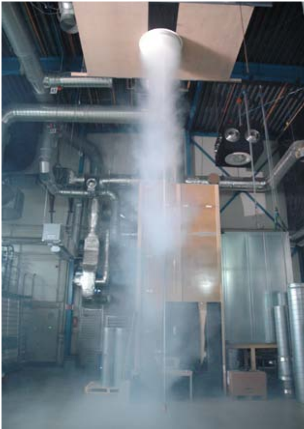
Fig. 4: Heating mode with air outlet volume flow rate of 695 l/s [2 500 m³/h] and \Delta\vartheta_H = +8 K from 8.2 m height
